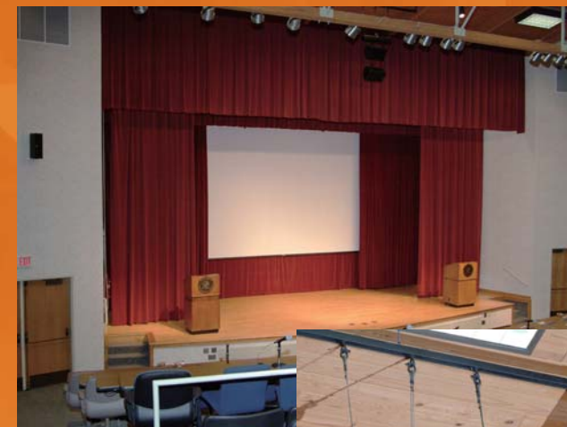
The Edith Macy Conference Center, Briarcliff Manor, N.Y. Boulevard Production Specialists Inc. designed and installed updated sound and video systems for the Center's 185-seat auditorium, dining area, and common area.
