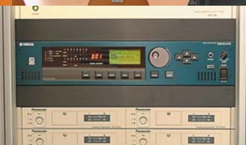
A DME24N is shown in the rack with a switcher. The number of channels provided by the switcher has been selected to match the size of the classroom or lecture hall.
