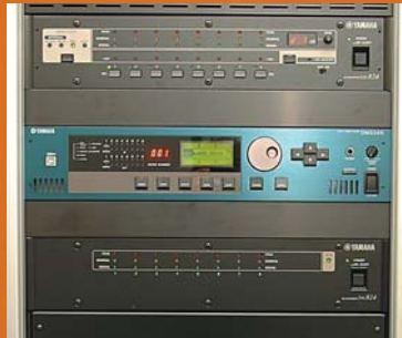
A DME24N, switcher, booster, and other gear in the equipment rack are operated from the touch-panel controller.
